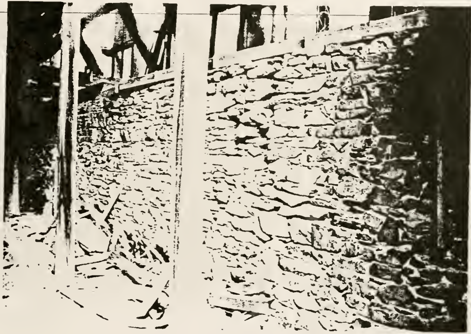
Figure 154. Interior of Arsenic plant (structure #59) showing detail of stone foundation wall, south end of eastern-most wall.
